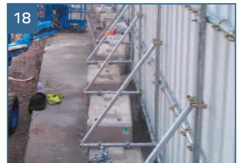
18 If required, the concrete blocks can be turned side-on and the installation process remains the same, however the tube lengths and spacing will change.
