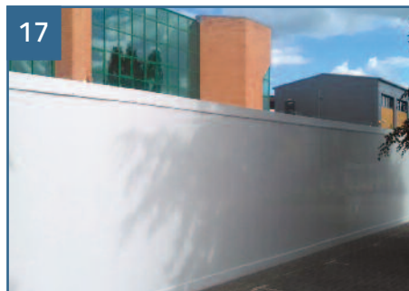
17 Trims are fitted with fixing screws to the top and bottom of the hoarding panels as shown.
