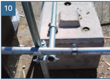
10 Once the first rail is secured, connect the next rail using a joint pin and secure in place using the Single Scaffold Fittings.
