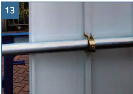
13 Connect the board to the frame at the centre line of the first board to the bottom, middle and top horizontal rails, using the Go Hoard clamps, as shown.
