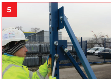
Attach Brace Plates to Post with M16 Coach Bolt Set (Ensure post is vertical & two bolts fix each plate).
