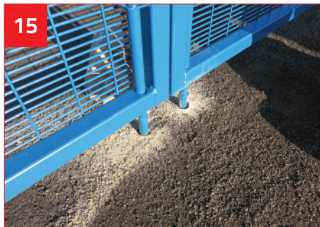
15 Drill holes to receive Drop Bolts when gate closed and open. (Install Ground Tubes where appropriate).
