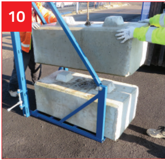
10 Place two Ballast Blocks on Support Base (Use Lifting Clutch for ease of positioning).
